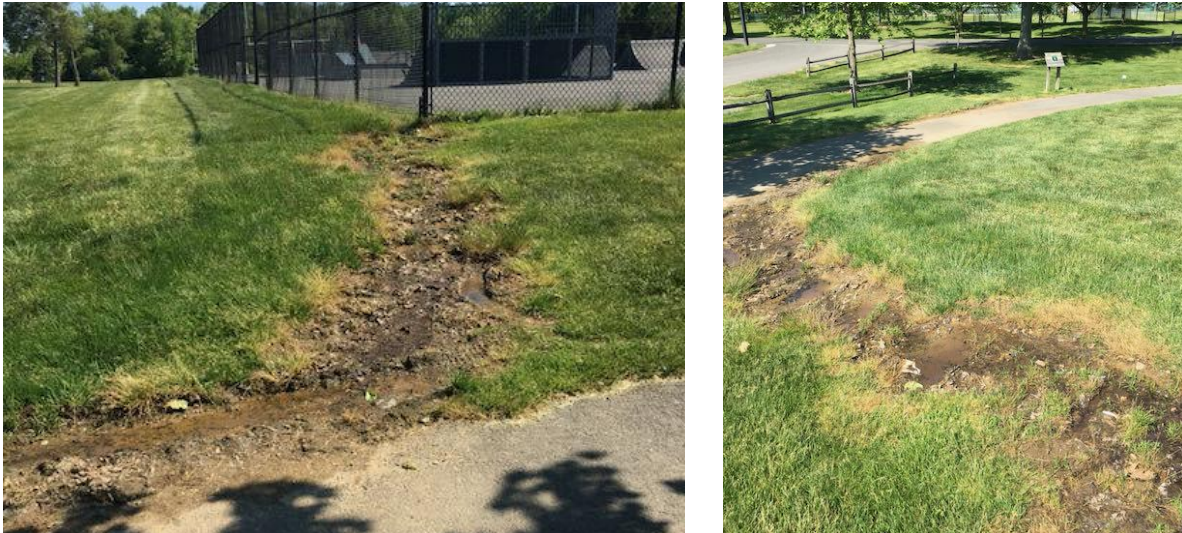
Figure 2: Erosion caused by water exiting porous material under the skatepark
